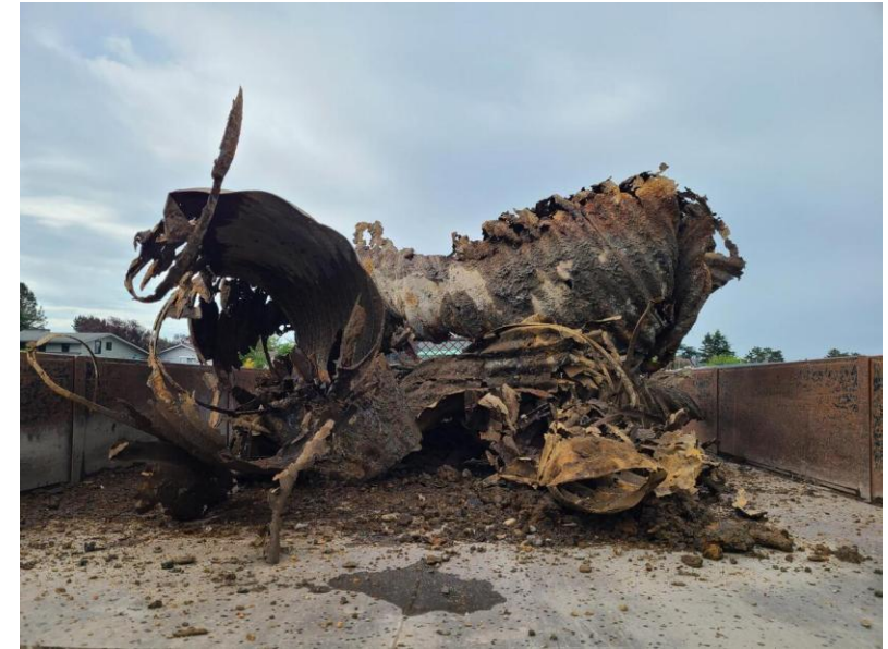
Aged, deteriorated corrugated drain pipe (Salish Lane)
