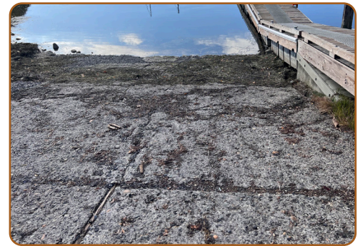
The existing ramp is more than five decades old, showing its age in spalled concrete and potholes.
