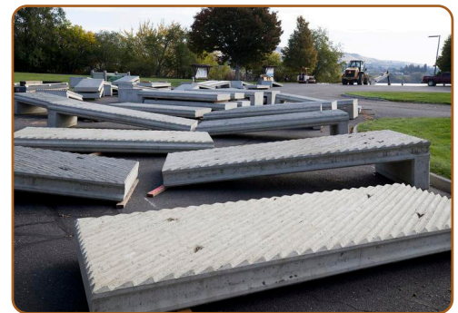
Precast concrete planks prepped for installation at the 2020 Confluence State Park boat ramp project in Wenatchee, WA. Source: The Wenatchee World
